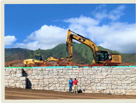
EVP Michele Kawahara and CEO/President Gary Fukuroku in front of the completed retaining wall on the February 25, 2021 site visit.
